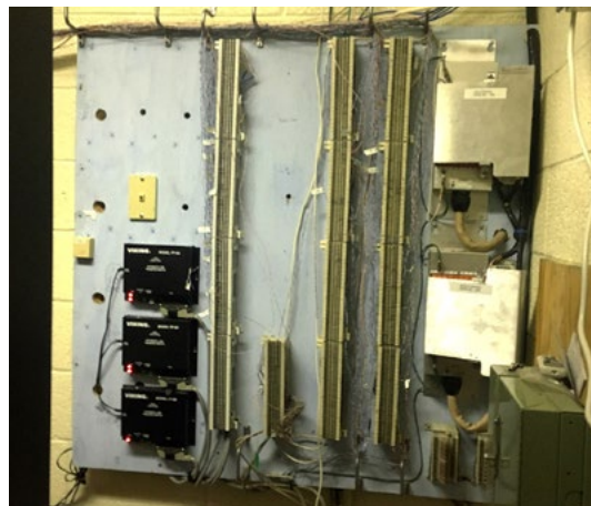
Main copper backbone distribution wall field in Elementary School MDF
